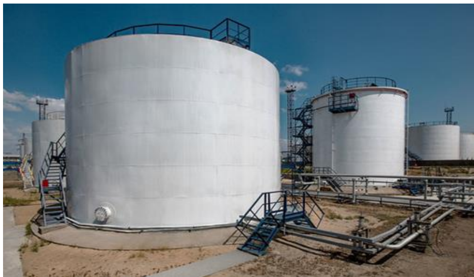
Figure 6. to white tanks - mixing park
