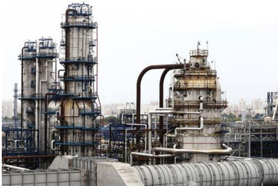
Figure 1. Primary processing unit for cleaning oil from water, salts, and sand
